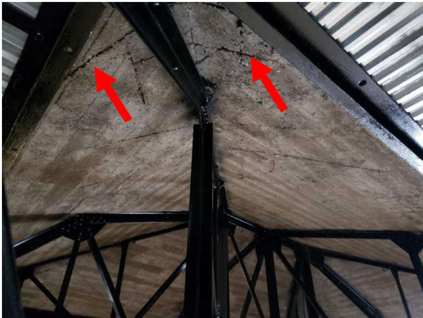
Figure 6. Underside of dome cap. The dark lines (red arrows) are embedded wood that Pishny noted have little to no concrete cover.
