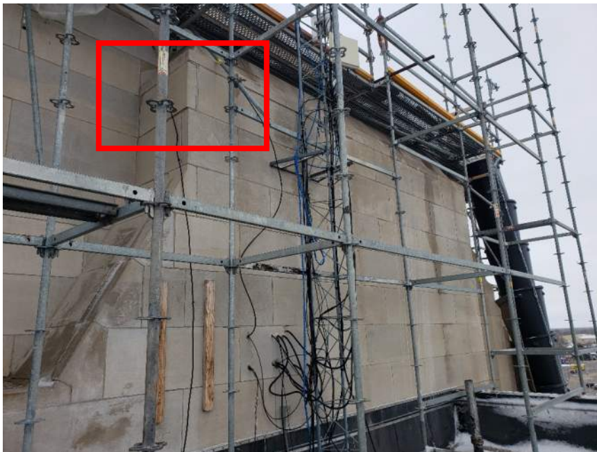
Figure 12. West elevation of the tower. See Figure 13 for an enlarged image of the offset corner stone boxed in red.
