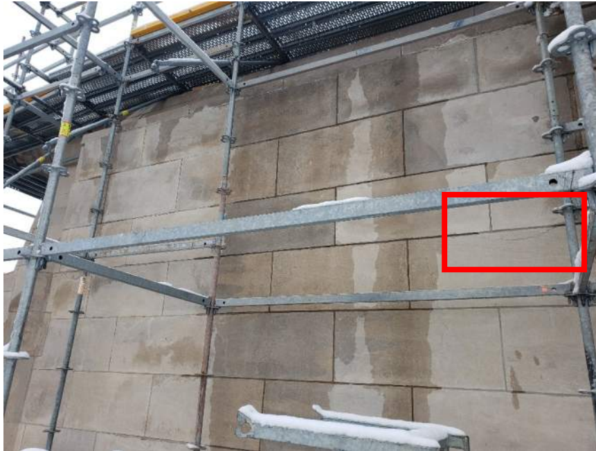
Figure 7. East elevation of the tower. See Figure 8 for an enlarged image of the “half-moon” stone crack boxed in red.
