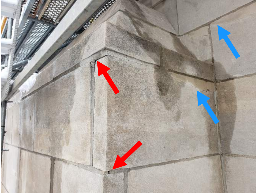
Figure 9. Locations of visible gaps at the stone mortar (red arrows) and "half-moon" patch repairs (blue arrows).
