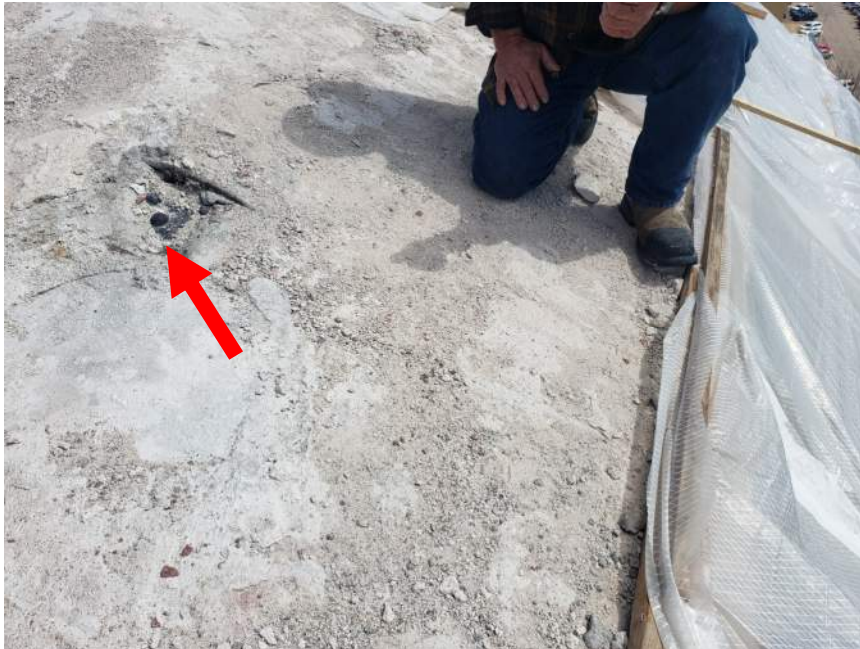
Figure 17. Southwest quadrant of the dome cap exposed. Slab reinforcing and rivets for the steel truss below were exposed at this location (red arrow).
