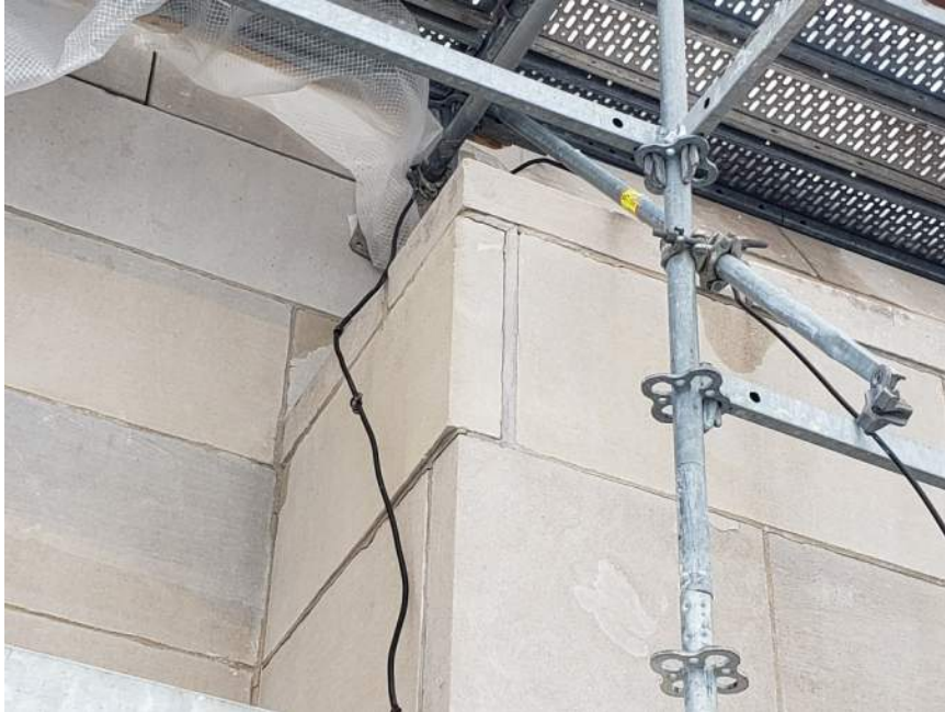
Figure 13. Enlarged image of Figure 12 showing a corner stone that is offset from adjacent stones. There are no large gaps or signs of distress in the adjacent mortar, suggesting that this stone may have been installed offset.
